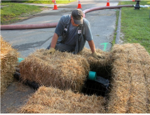
Leachate Discharge from Dewatering Containment
